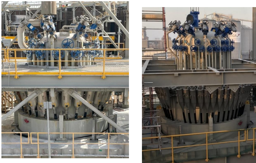
Figure 8. Hydrocyclone distributors. (a) primary stage, (b) seed stage. One of three clusters each.
